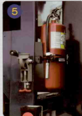
5. Fire extinguisher - 20lbs
